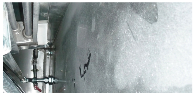
View inside an exhaust plenum fitted with UV-C lamps after several weeks of use
