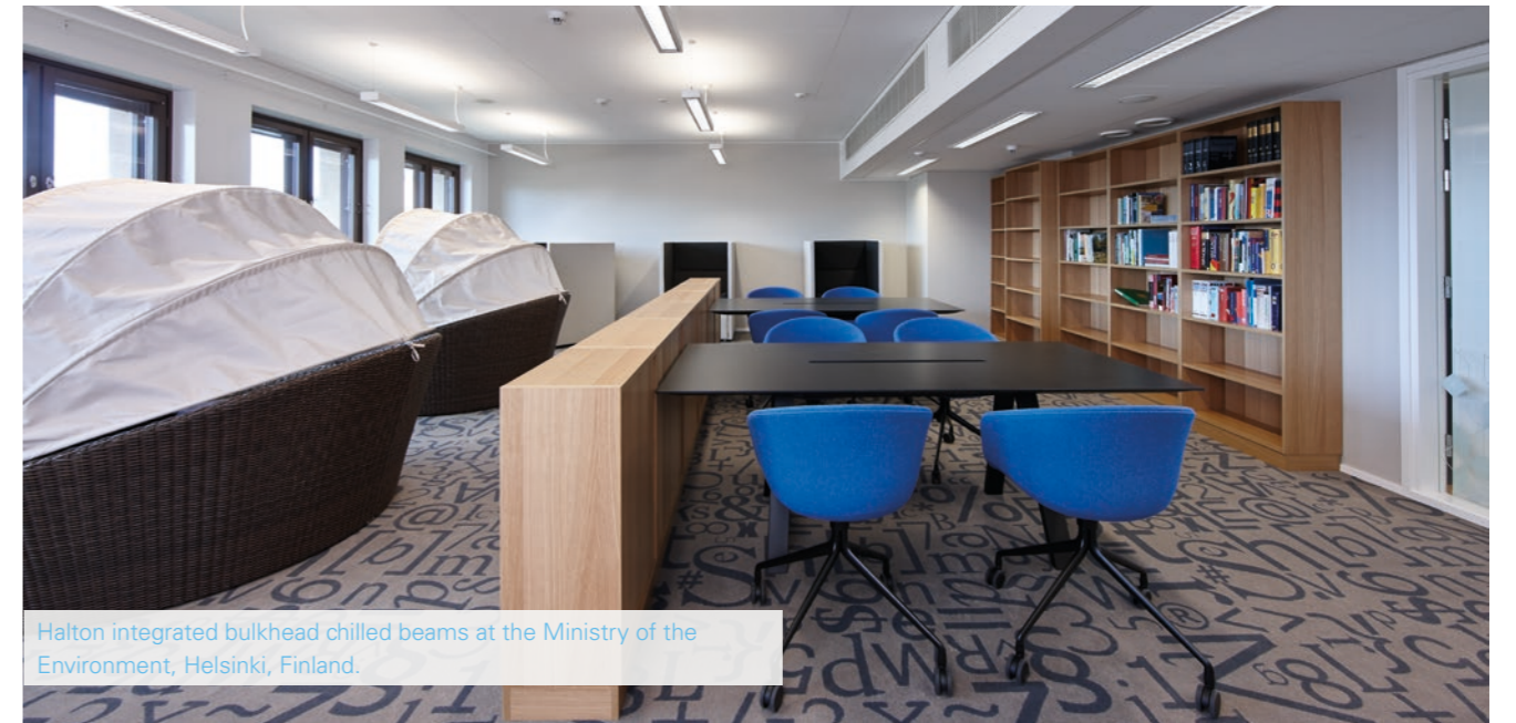
Halton swirl comfort active chilled beams with Halton Vario system at the Ministry of the Environment, Helsinki, Finland.
