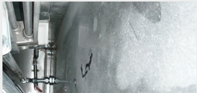
View inside an exhaust plenum fitted with UV-C lamps after several weeks of use.
