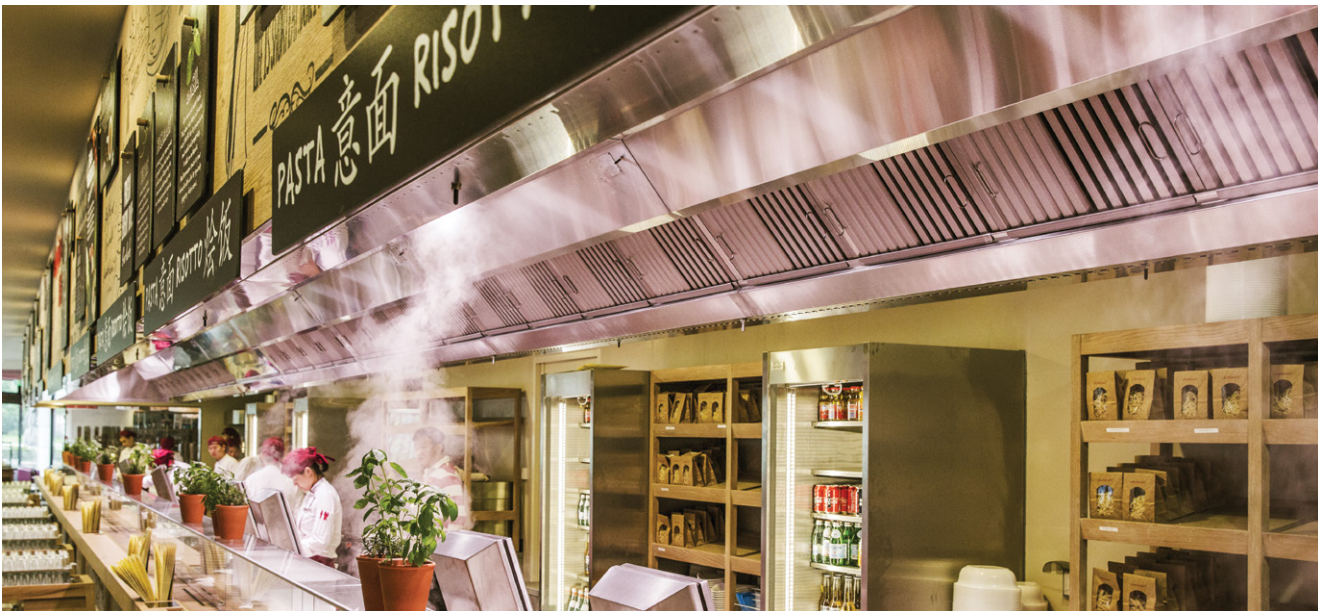
Vapiano Restaurant (Shanghai, China)
